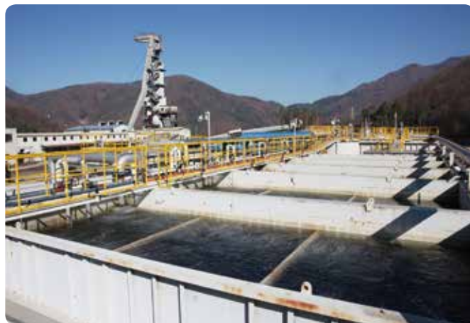
High1 Resort's Advanced Water Treatment Plant
