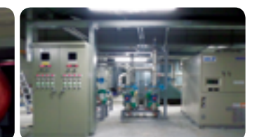
Waste heat recovery equipment
